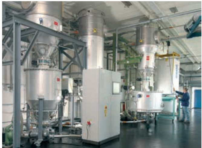
Figure 10 Pneumatic suction conveying system in the Handling Pilot Plant in Hanau
